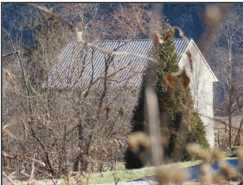
Figure A-12. CRA 1. South and west elevations of the modern house, looking northeast.
